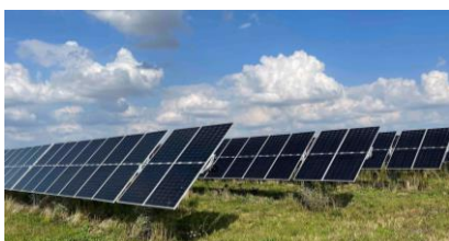
Invenergy's Hardin Solar Energy Center, located in Hardin County, Ohio.
